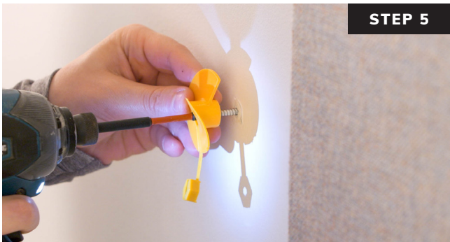
Screw Rotofast Standard Anchor to wall at marked location. Make sure the anchor spins on the shaft of the screw but does not wobble.
